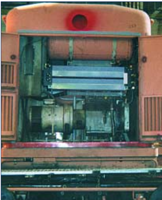
Position of the domnick hunter Adsorption dryer installed by DB cargo, Chemnitz, Germany.
