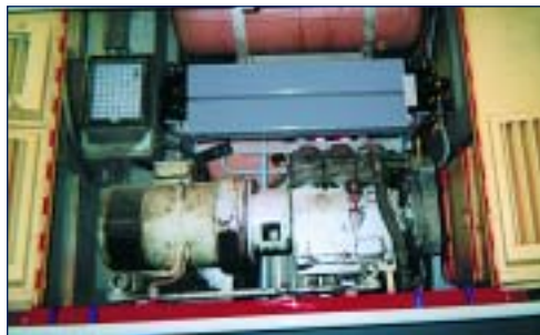
Air receiver, domnick hunter Adsorption dryer, Compressor.
